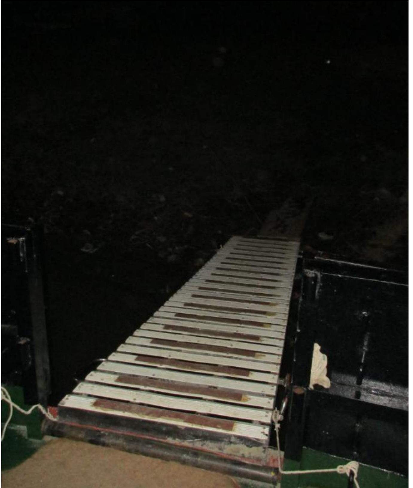
Example D: The gap between gangway and platform is a potential trip hazard.
